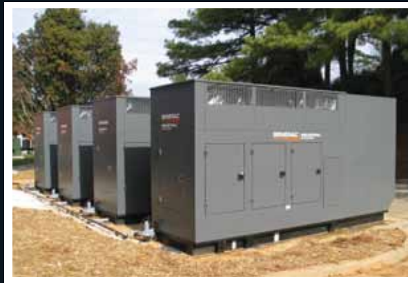
The gaseous-fueled Generac generators in this telecommunications switching application are installed in parallel specifically to provide redundancy.
