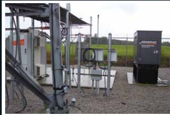
Cell sites like this one benefit from the rugged reliability of Generac diesel-fueled generators with large base tanks.
